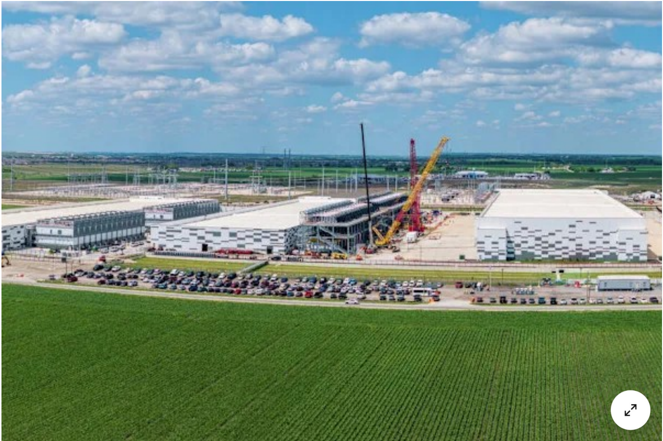
Aerial view of the Skybox Power Campus under construction in Hutto, Texas near Austin. Project plans call for four million square feet and 600 megawatts power at the facility. (BackyardProduction/Getty Images)
